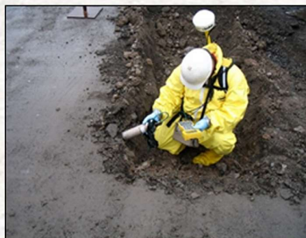
To the right, Northwind tests soil for hazardous contaminants on a remediation project
